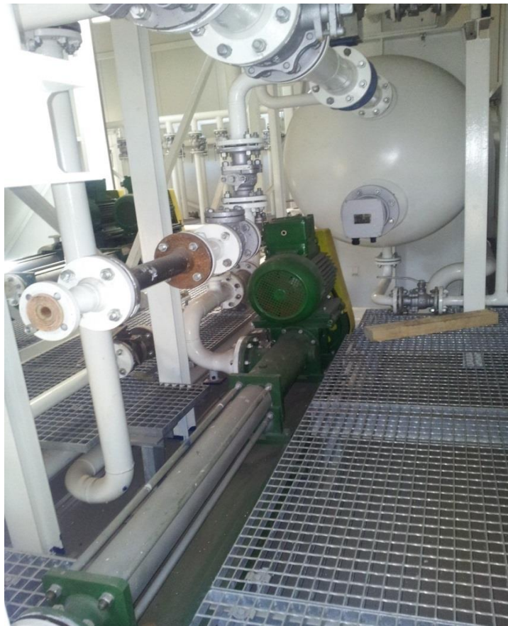
GPEO-7,5x24 mounted in skid.
