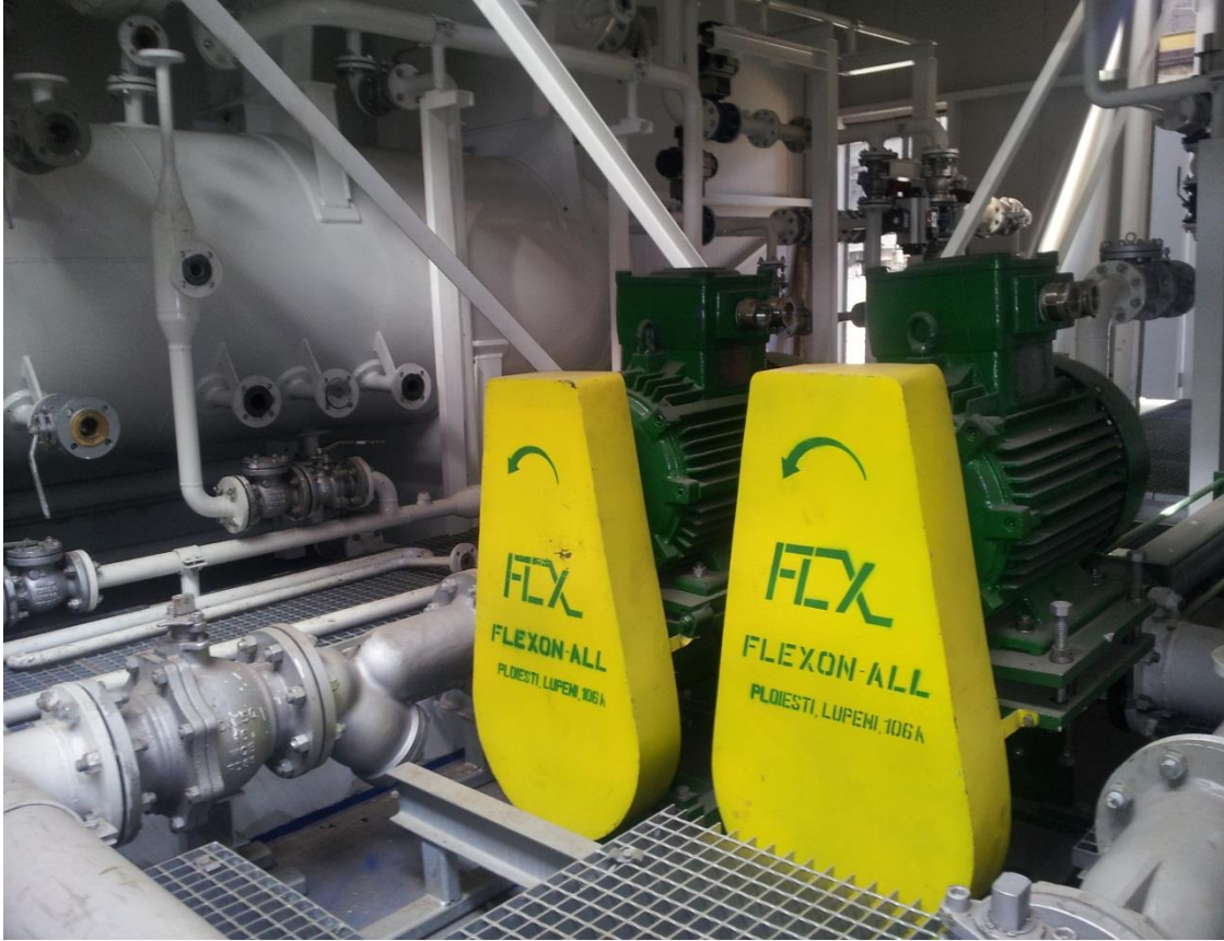
GPEO-16,5x24 mounted in skid.
